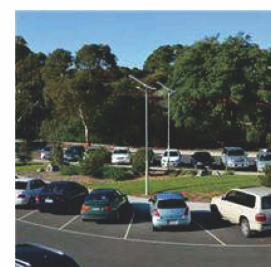
Square & Parking Solar Lighting
